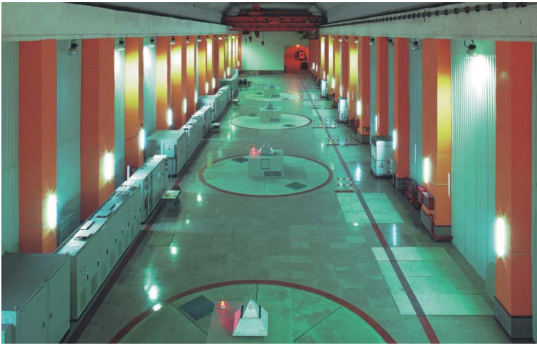
Machine Hall at 400 MW Vishnuprayag Power Station, Uttarakhand
