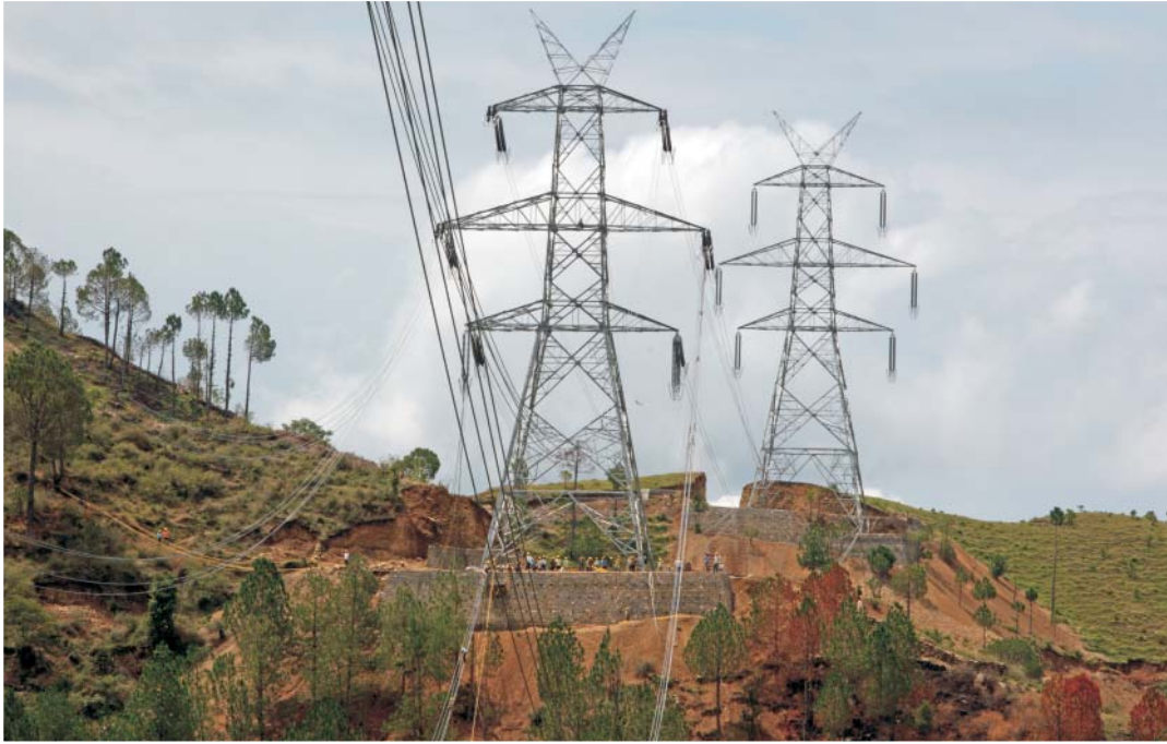
Transmission line of Jaypee Powergrid from Wangtoo to Abdullapur, Himachal Pradesh
